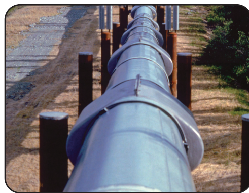
Figure 58. The Trans-Alaska Pipeline
