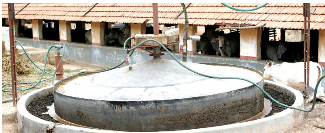
Fig.3.11-Biogas (Gobar gas) plant
