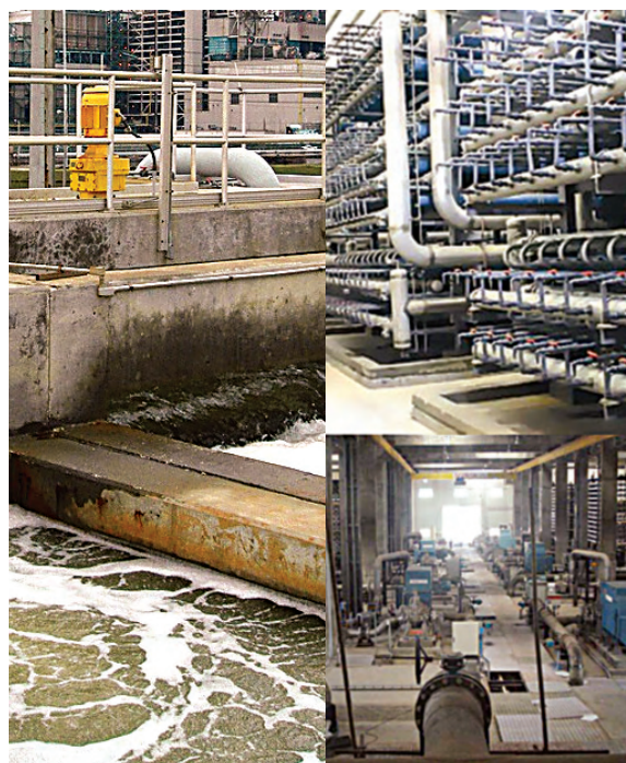
Fig. 2.12. The Desalination Plant at Minjur, Thiruvallur Dt.,
